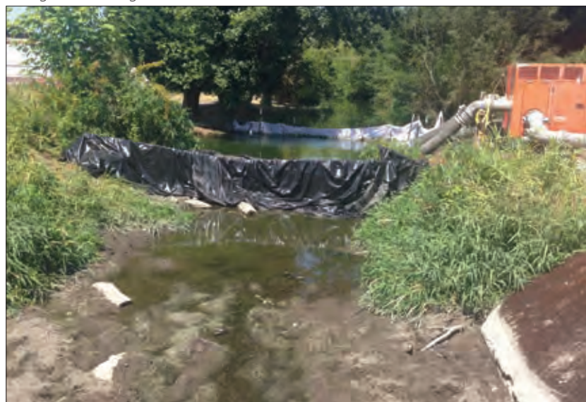
Figure 28. This channel was dewatered to replace a downstream culvert. Water was pumped around the project area to allow for access. Mussels were salvaged and relocated before the area was dewatered, during the fish salvage, and during the final drawdown.
