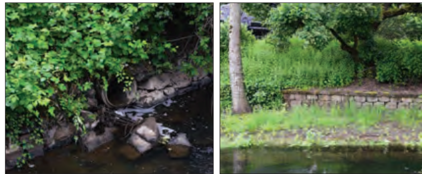
Figure 24. Left: Retaining walls that cover banks and are built up from the streambed limit mussel habitat. Right: When walls are set back from the water's edge, a larger area of natural shoreline is retained, which can provide better mussel habitat.
