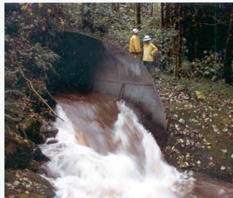
The historic culvert had a firehose effect on downstream habitat, flushing out spawning gravels.
