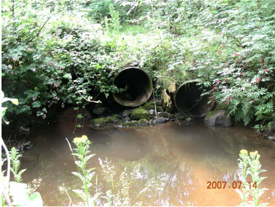
Photo 14. Three Culverts on Spilde blocking juvenile migration
