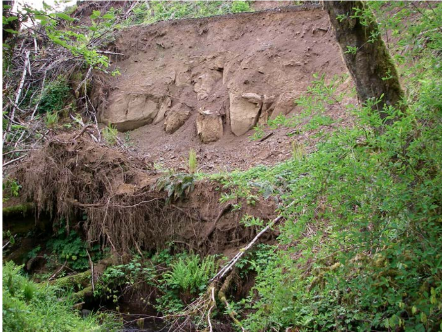
Photo 2. Road failure on Buttermilk Creek
