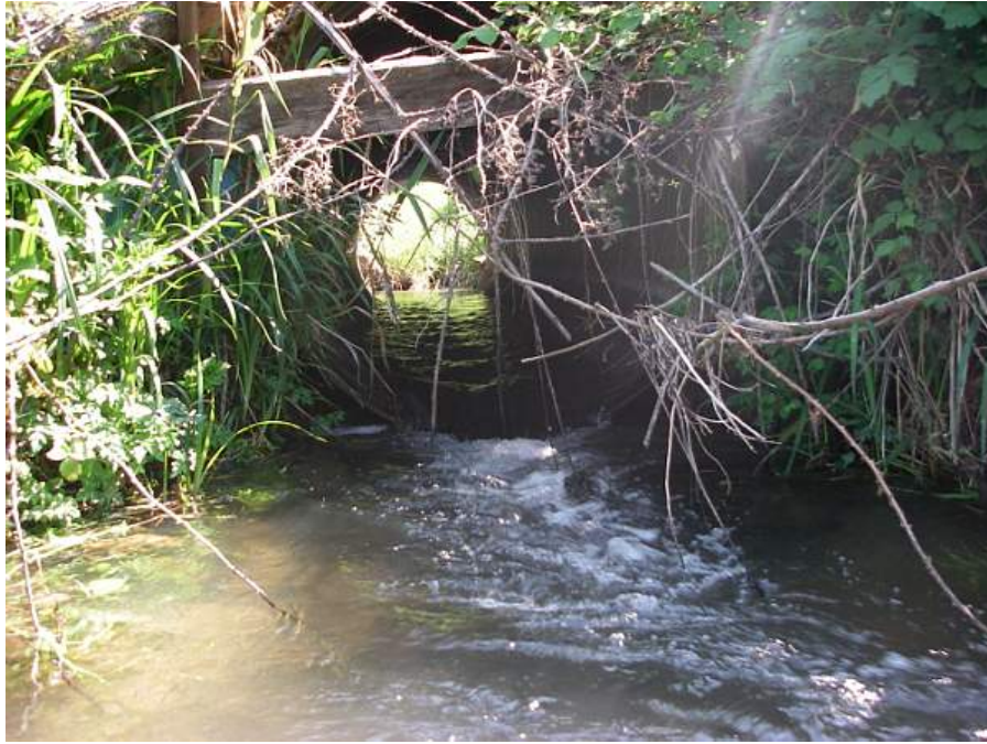
Photo 8. Second culvert on Young Creek with rusted bottom, flow beneath.
