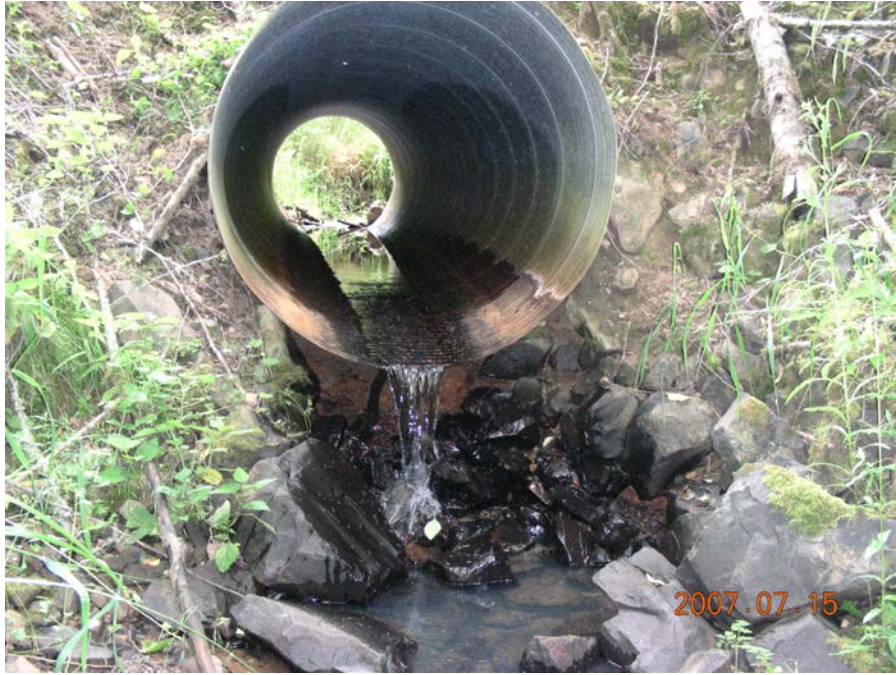
Photo 15. Coho found above this 16" drop onto riprap. 1 st pipe above county road on Spilde Creek
