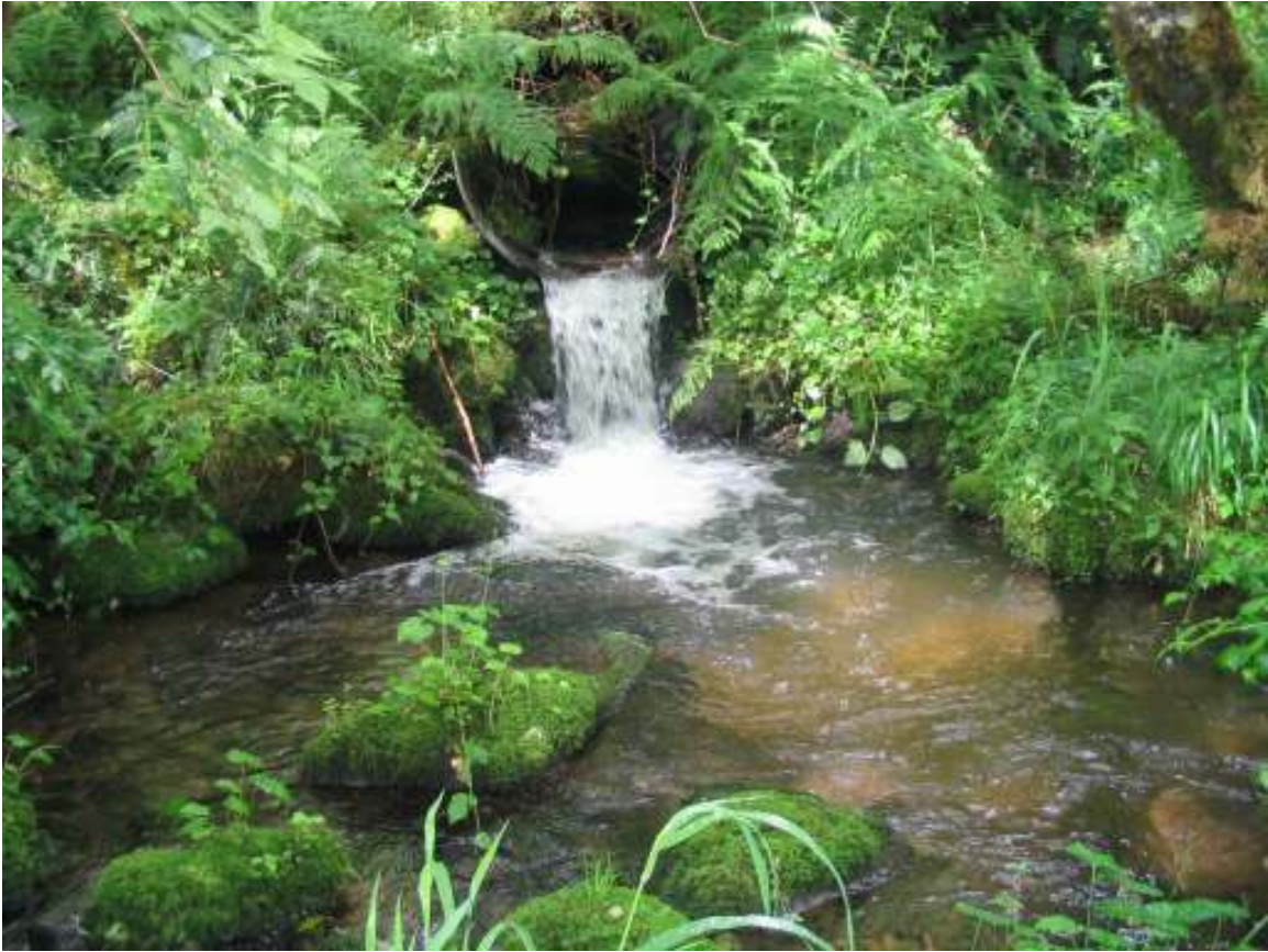
Photo 11. Perched culvert on Trib E; definitive juvenile barrier.
